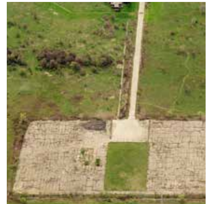
The far east parking lot is in very poor physical condition.
